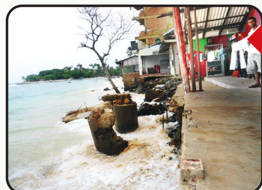
Degradation of coastal environment due to unauthorized constructions without obtaining coast conservation permit.
