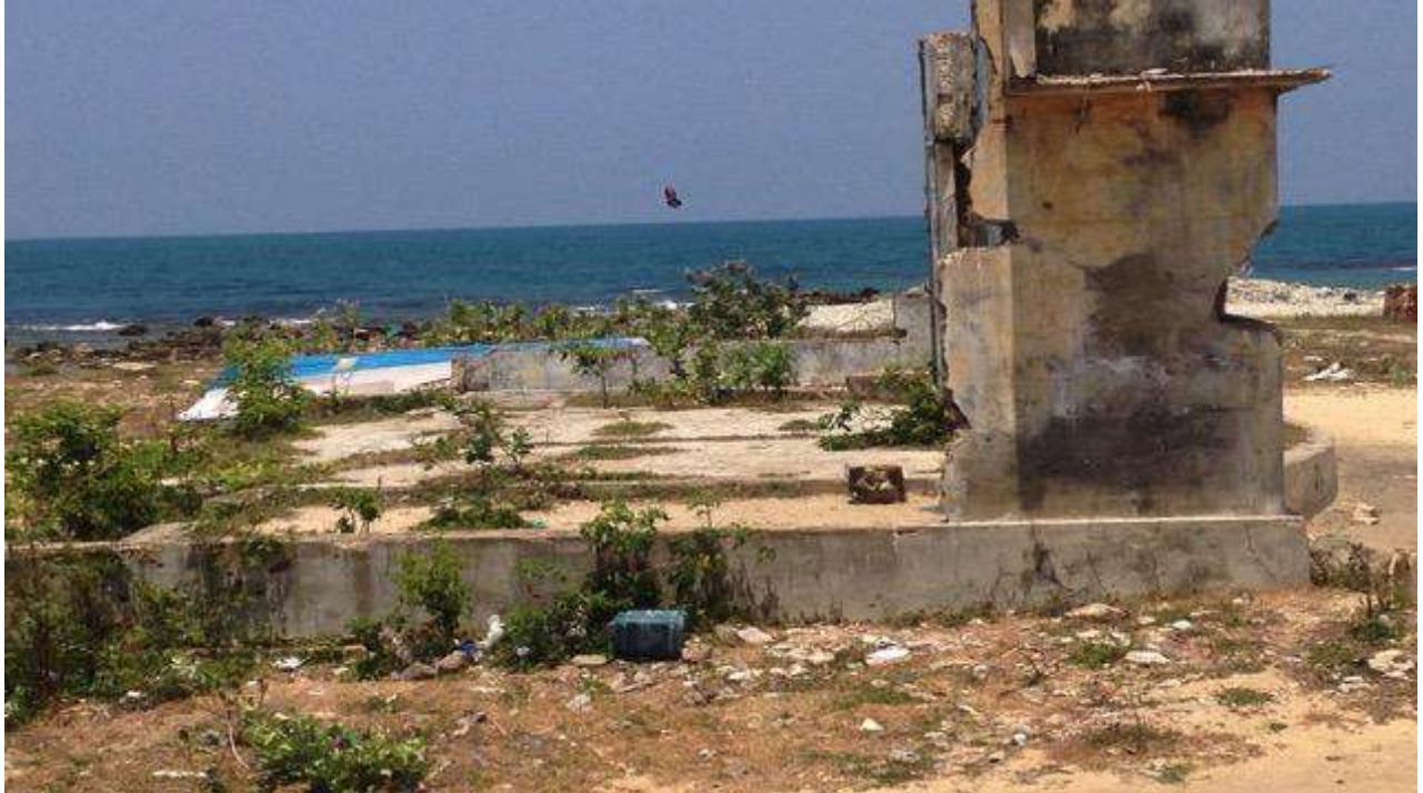
Fig. 9. Abandoned and damaged Natarajar Stadium with emerging vegetation
